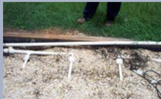
Failed sand filter
